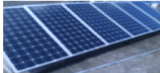
Figure 6. 1.2 kW p PV array at rooftop
