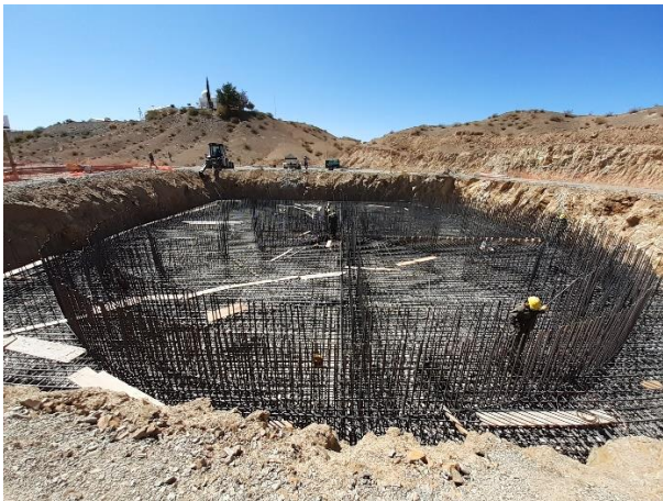
Figura 6. View of the work, the reinforcement of the foundation slab and the emerging cylinder can be seen.
