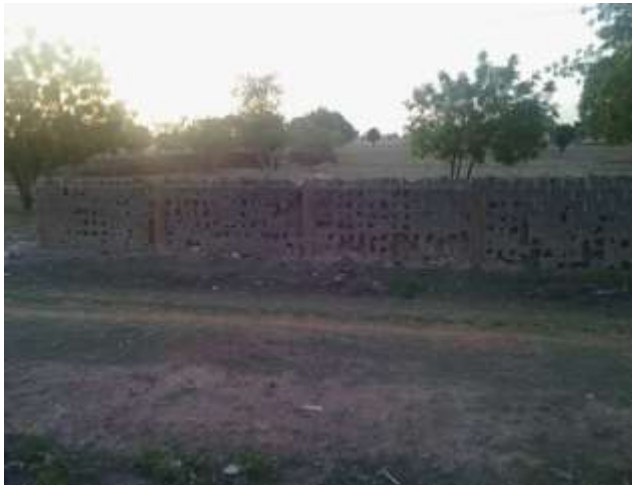
Plate 2: Wall built with poor Quality Blocks
