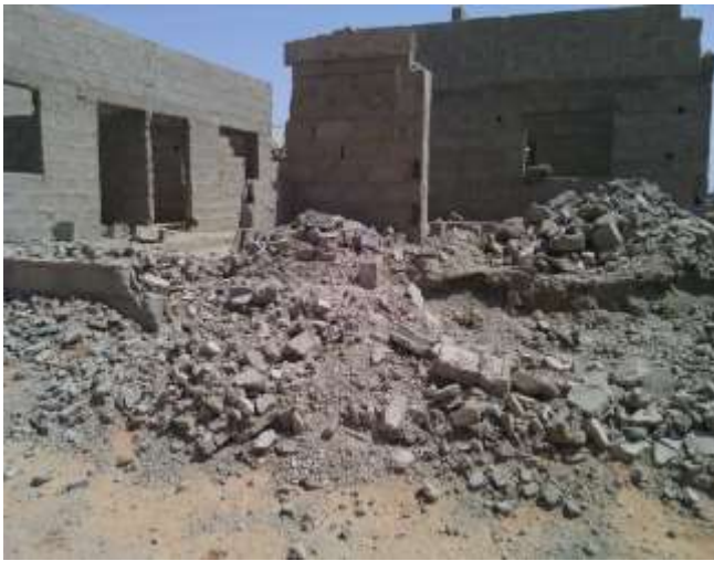
Plate 1: Collapsed Residential Building under Construction at Barhin Quarters
