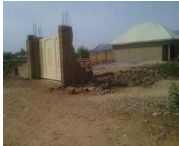
Plate 5: Collapsed block wall fence around Residential Building
