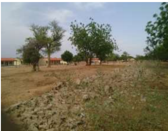
Plate 3: Collapsed block wall fence around public School
