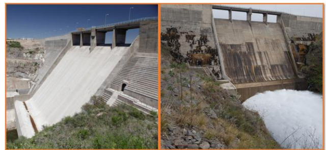
Figure 1. Photos. The dam presents the day of the inauguration, and five years later. There is upwelling of water on the wall waters down by leaks
