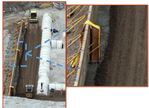
Figure 4. Photos. Shows the lack of detail in the placement of the gasket water-stop.
