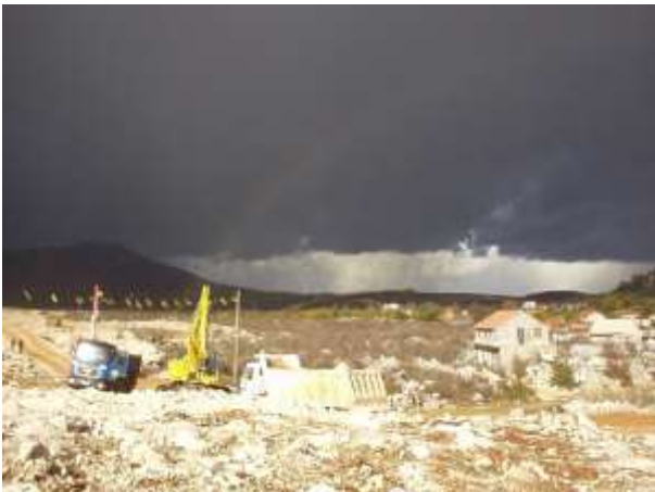
concrete underground tanks, which are also one of the problems for blasting.
