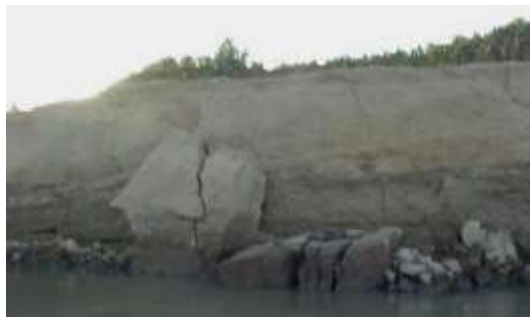
Figure 17. Bank Erosion in the Main Nile [24].
