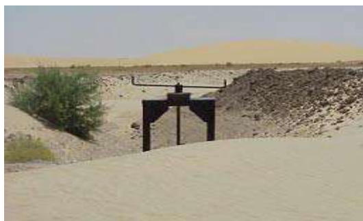
Figure 18. Irrigation Canal Buried with Sand Dunes in the Northern State – Sudan [24].
