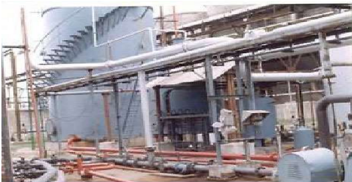
Figure 4 Biological Hydrogen Production Plant set up by MCRC, Chennai
