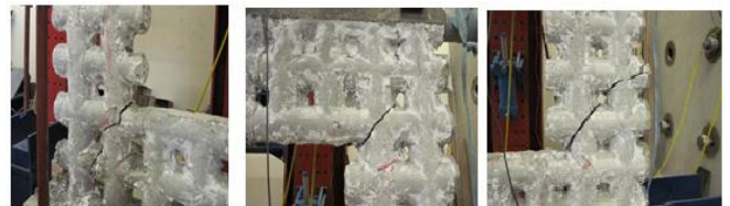
Figure 4 Cracking of SW1, lower left corner (left), upper top corner (center), lower right corner (right)
