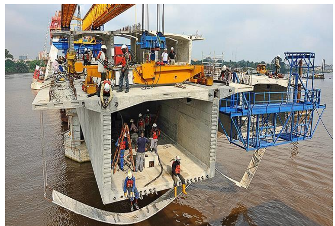
Figure 3.2. Deck cross section and cantilevered techniques construction of Lekki Bridge (Julious Berger Plc, 2013)
