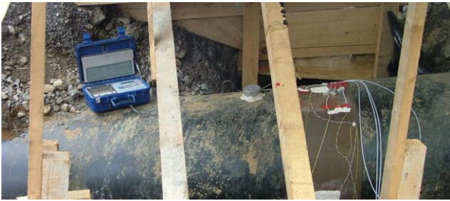
Figure 2. Measurement setup on the oil transmission pipeline [10]
