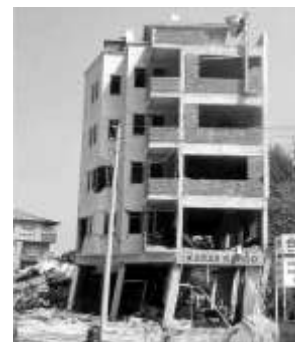
Fig. 1 Formulation of soft storey mechanism during Turkey earthquake, 1999 (Sezen [8])
