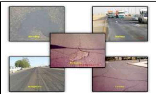
Figure # 1; Deformation of asphalt pavements
