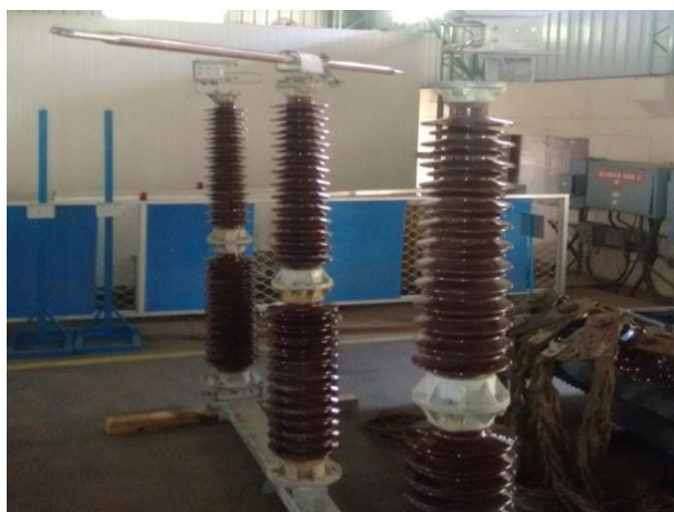
Fig. 5 A View of Movable assembly for 220 kV Isolator
