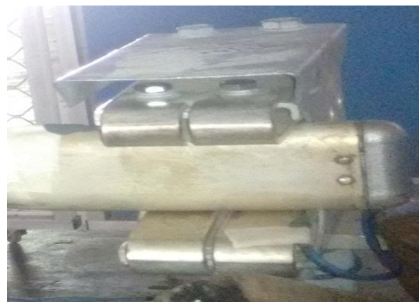
Fig. 3 A View of Fixed assembly for 66 kV Isolator
