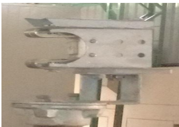
Fig. 6 A View of Fixed assembly for 220 kV Isolator
