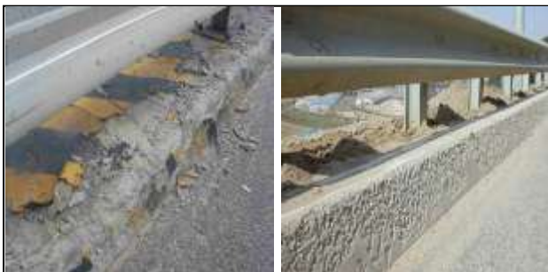
Figure 1. Damages at road facilities due to chloride-based deicers
