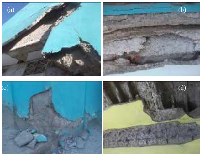
Fig. 3. Damages observed in situ: a) cracks and large expansion of mortar; b) concrete spalling with white coating; c) expansion of concrete and materials loss; d) concrete transformed into mush
