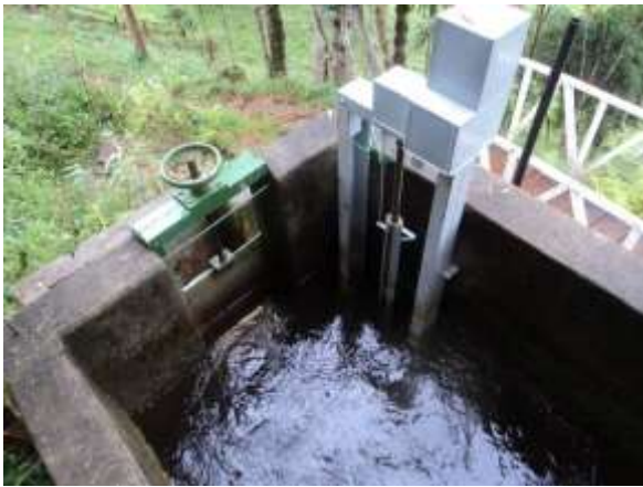
Figure 8: The floodgate at right is actuated by a DC 24[V] motor located at the top. This voltage is supplied by batteries. The entrance of the pipe is located under water.
