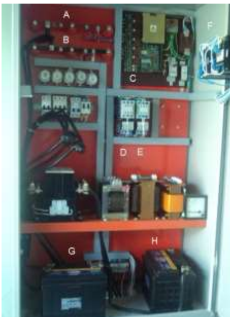
Figure 12: Power house cabinets (Legend: A - positive bar; B - negative bar; C - Semikron MP410T board; D - K1 contactor for floodgate descent; E - K2 contactor for floodgate rising; F – under-voltage and overvoltage relays; G and H - batteries).
