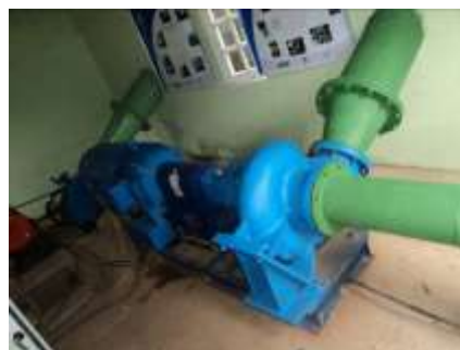
Figure 2: Pump as Turbine/Induction Generator group(Induction motor nameplate data: 45[kW], 60[Hz], 220/380/440[V], 1780[RPM], power factor: 87%, efficiency: 93.1%, manufacturer: WEG)
