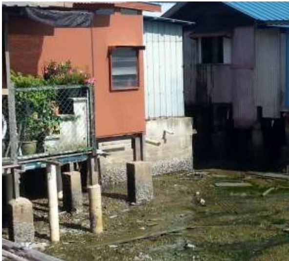
Figure 5 Human waste floating on the water surface
