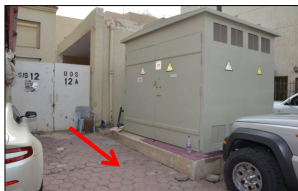
Fig. 4. Qortuba substation no. 12 indicating highest magnetic field levels
