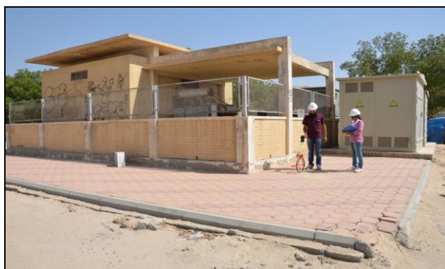
Fig. 1. Measurement taken using LINDA wheel around the electrical transformer.
