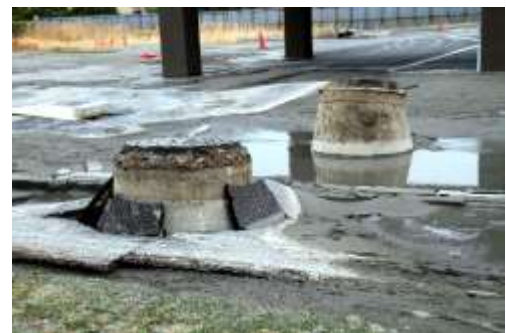
Figure 1 Manhole protruding by liquefaction
