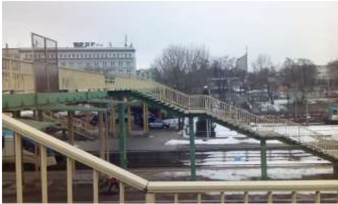
Fig. 1. The view from the bottom of the stairs structure of a footbridge in Bielsko-Biala - Source: own
