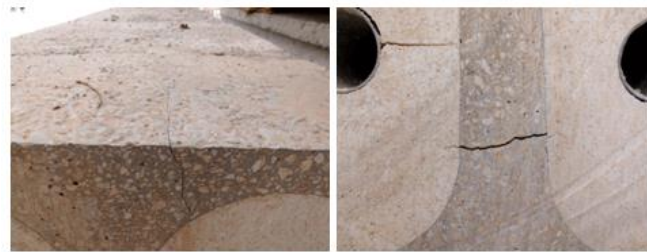
Figure 7. Longitudinal and horizontal cracks in SCC HCS units.
