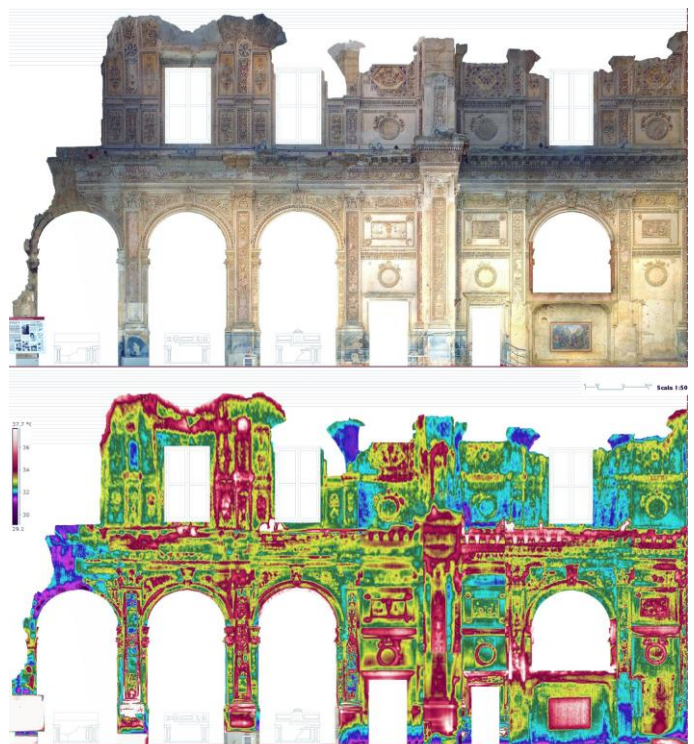
Figures 1-3. Santa Margherita di Belice (Agrigento), maps of the restoration project concerning the degradation analysis on thermal anomaly.
