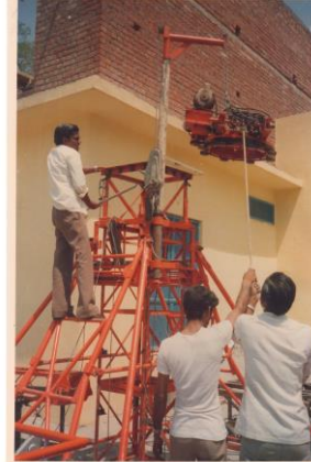
FIG.05 MINNI CLIMBING CRANE UNDER ERECTION. THE ASSEMBLY OF RING GEAR AND PLATFORM CHASIS (WEIGHING ABOUT 170 Kg.) IS BEING LIFTED UP WITH THE HELP OF PIVOTED POLE HOISTING GADGET.
