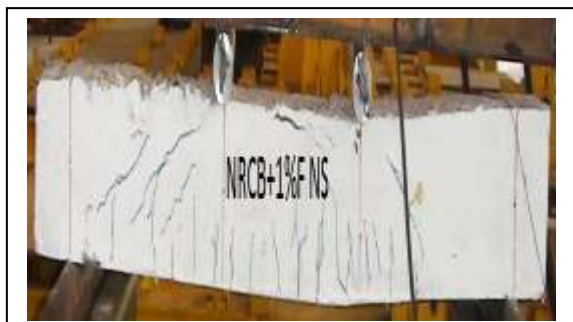
Figure 9 RC beam with full shear reinforcement, 10kg/m³ kenaf fiber
