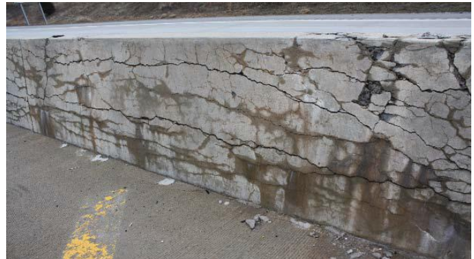
Figure 2. Barrier wall exhibiting ASR deterioration.
