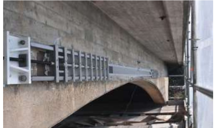
Figure 6. Strengthening of The Nossan bridge in Sweden with two laminates, pre-stressing force of 100 kN in each laminate.
